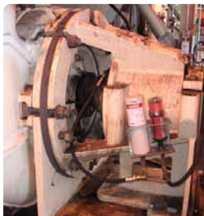
Equipment: Metso pump perma Star Vario MB02-C with BC30 Lubricator: perma Star Vario MB02-C with BC30 Bracket: K230C Install Kit: K230C Ref #: PUMP11
