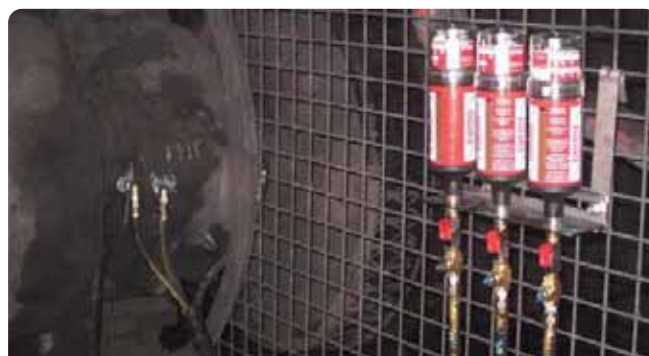
Extreme levels of contaminants shown here on a conveyor pulley bearing in the coal industry. Remote mounted perma Star Vario lubricators are providing lubrication and protection around the clock.
