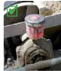
perma Futura providing bearing lubrication and seal purge to prevent the ingress of contaminants on a snub pulley bearing.
