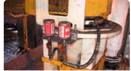
Equipment: Metso sump pump perma Classic MB02 with BC30 Lubricator: perma Classic MB02 with BC30 Bracket: K230G Install Kit: K230G Ref #: PUMP03
