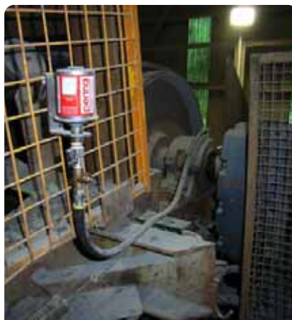
perma Classic remote mounted to the outside of a conveyor safety cage in the quarrying industry, providing safe access for lubricator inspections and servicing.
