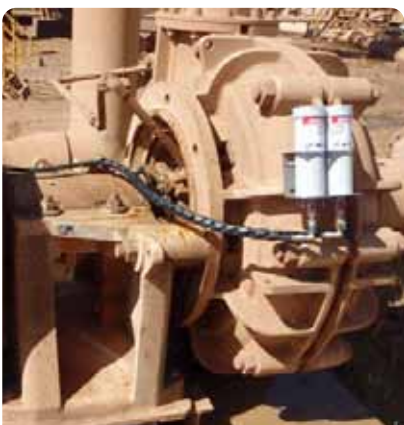
Equipment: Warman pump perma Star Vario MB02-C with BC65 Lubricator: perma Star Vario MB02-C with BC65 Bracket: K265C Install Kit: K265C Ref #: PUMP10
