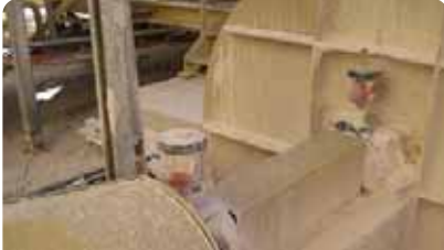
Lubricator: perma Futura Bracket: Direct Ref #: FAN01
