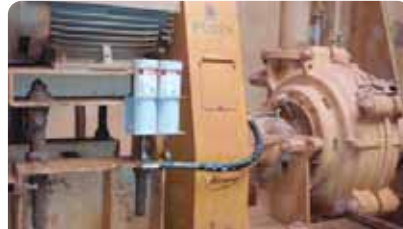
Equipment: Warman pump perma Star Vario MB02-C with BC30 Lubricator: perma Star Vario MB02-C with BC30 Bracket: K230C Install Kit: K230C Ref #: PUMP08
