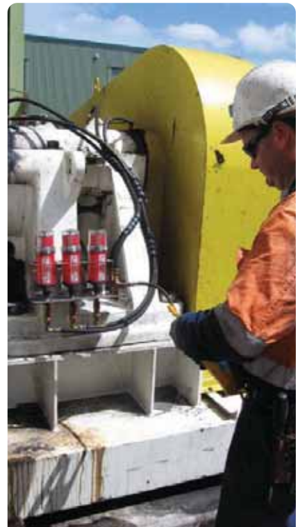
perma Star Vario lubricators remote mounted using a K365C2M installation kit. This kit facilitates the relocation of all (5) grease points for the pump to a safe to access location. The top of this pump barrel is at head height.
