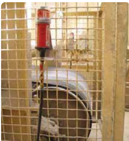
perma Star Vario lubricator remote mounted to a conveyor pulley bearing using a K1CH installation kit. Access is safe and the safety cages can still be easily removed if required during maintenance shuts.
